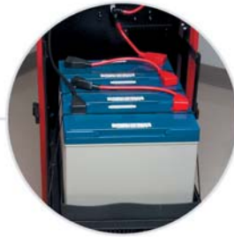
Maintenance free 140 ah AGM batteries
