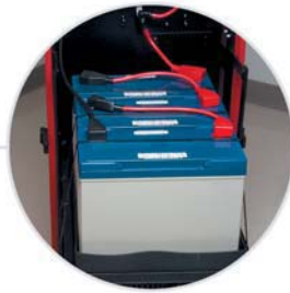
Maintenance free 140 ah AGM batteries
